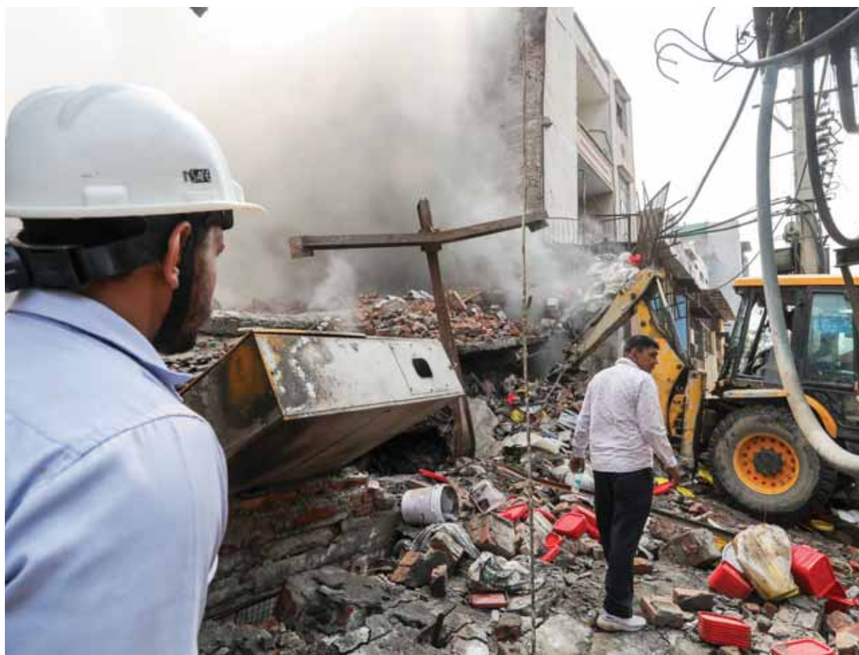
Debris of a factory building that collapsed due to an explosion following a fire at Bawana industrial area in New Delhi on Saturday
