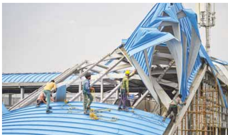
Workers repairing damaged roof of the New Ashok Nagar RRTS station in New Delhi PTI
